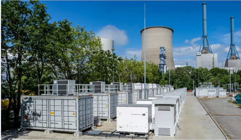
Figure 3: Battery storage system in Lingen and Werne, Germany (Source: RWE, reproduced with permission)
